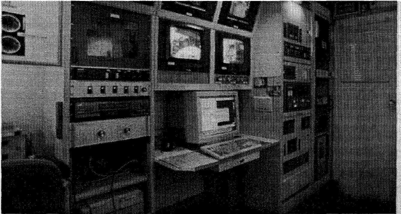
Figure 11 shows the WIT control room and operator's workstation.
