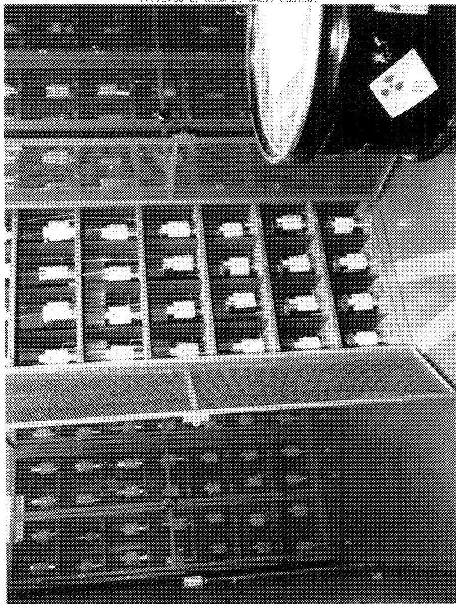
PPF/2736-Z, Room 2, Shelf Cubical
