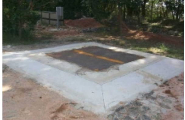
Figure 15 – Concrete and SS platform
