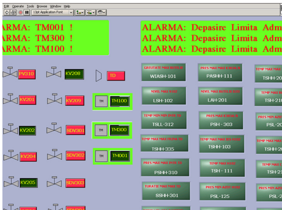
Figure 5: Monitoring station - Alarm parameters
