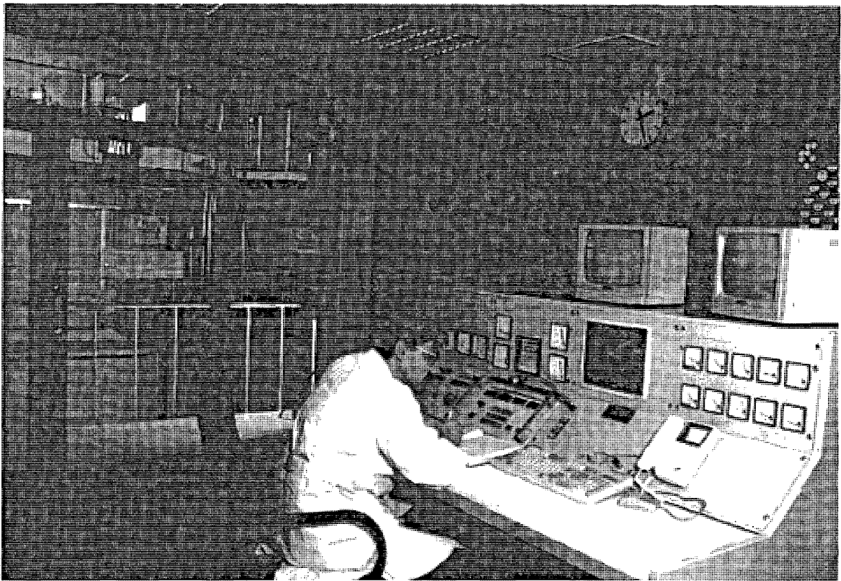
Fig. 2 TRIGA's Control System
