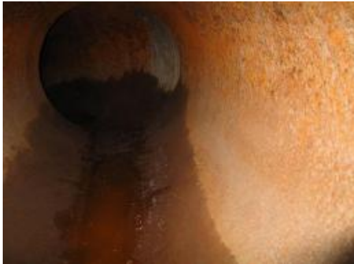
Figure 2 The pipeline before refinement from corrosion and sediment products
