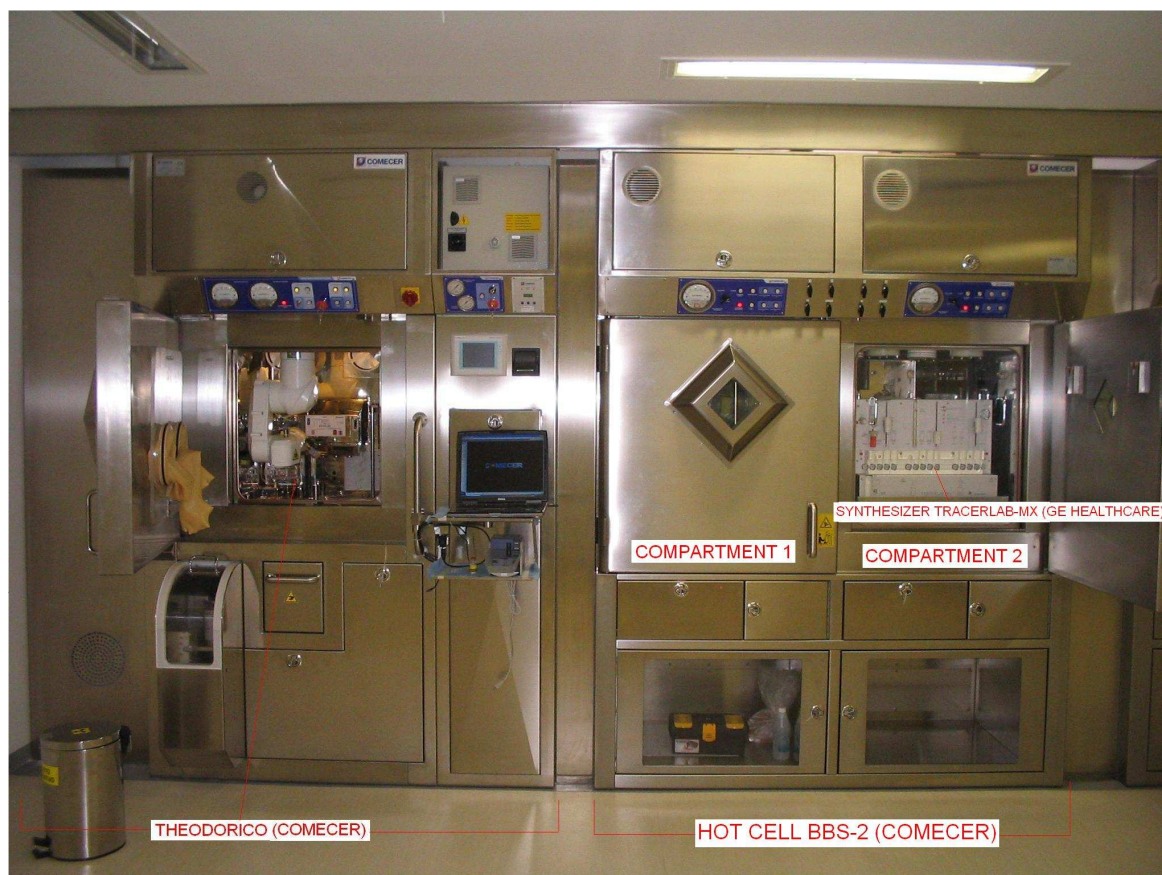
Figure 1. General view of the THEODORICO and hot cell BBS-2 (COMECER). Inside one of the 2 compartments of the BBS-2 is shown 1 of the synthesizers TRACERLAB-MX from GE HealthCare.
