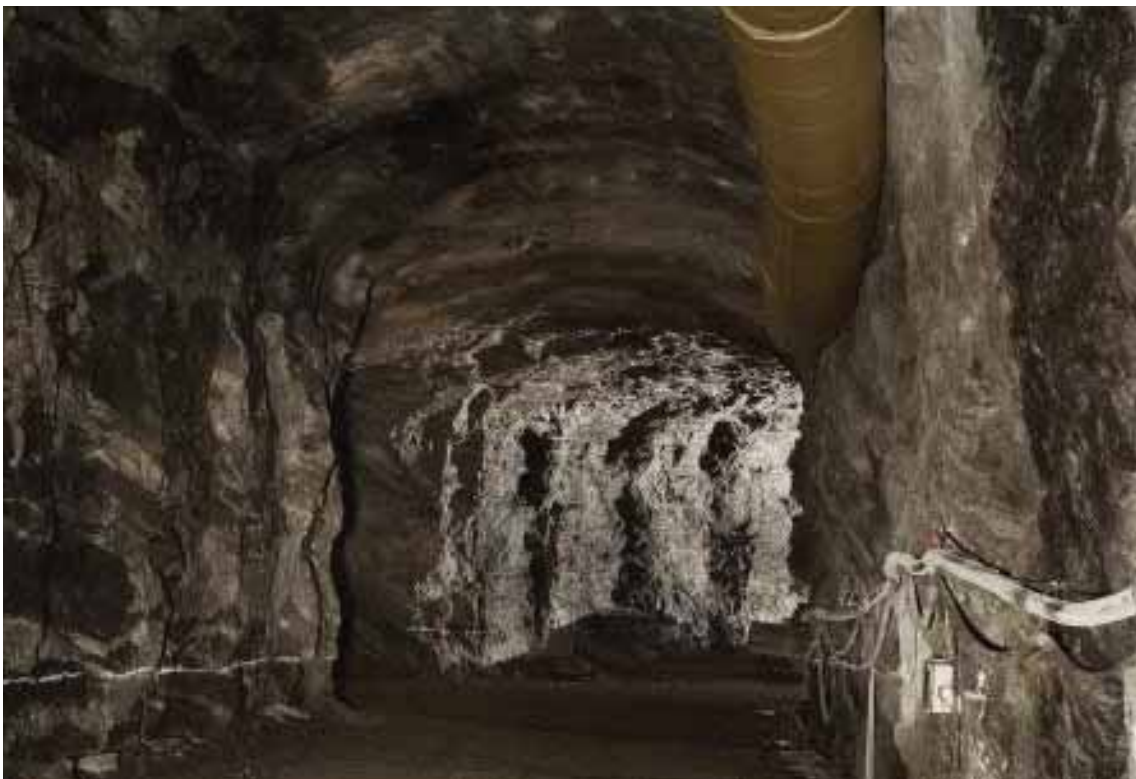
Figure 2. A section of the ONKALO access tunnel at Olkiluoto showing the extreme lithological heterogeneity which is characteristic of many parts of the Olkiluoto bedrock(Photo: Posiva).
