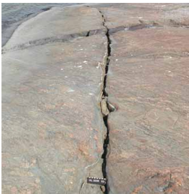
Figure 16. A very long fracture cutting through poorly foliated migmatitic gneisses on a shore outcrop near Olkiluoto (Photo 2006-63.1A from the Appendix "Outcrop Photographs" in Lindberg 2007, scale bar 15 cm). Towards the waterline the joint intersects the mafic dyke shown on page 17. Post-glacial movement on this joint of 2-4 cm (height difference of the glacially striated surface on either side) cannot be excluded (see Pere 2009, p. 3 and Fig. 3).
