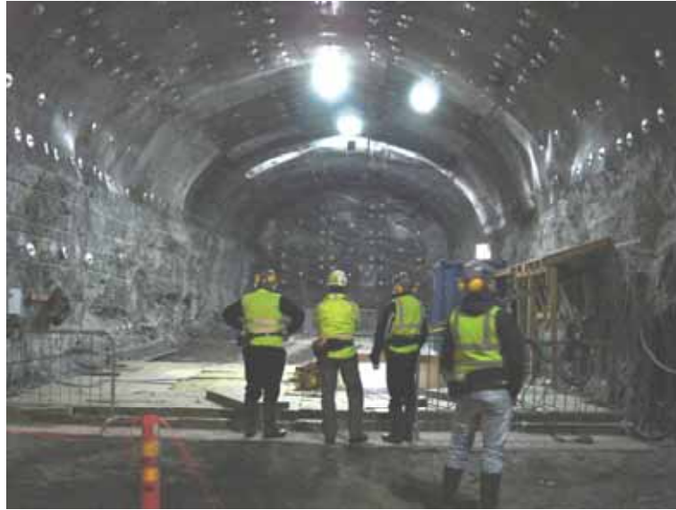
Figure 2-1. The rock mechanics niche in the ONKALO from which the ONK-PP259 drillhole cores were obtained. The niche is excavated in diatexitic gneiss, veined gneiss and pegmatitic granite.
