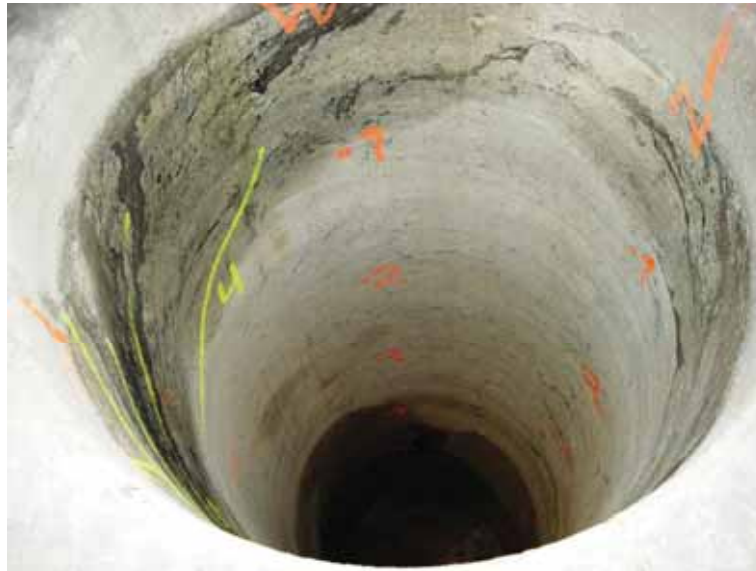
Figure 2-3. The ONK-PP259 vertical drillhole was drilled on the centreline of this \varnothing 1.5 m hole, i.e. before the hole was reamed.
