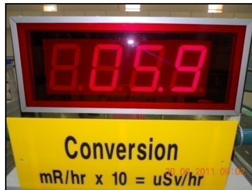
Figure 7: Water level monitor at the Pool Top
