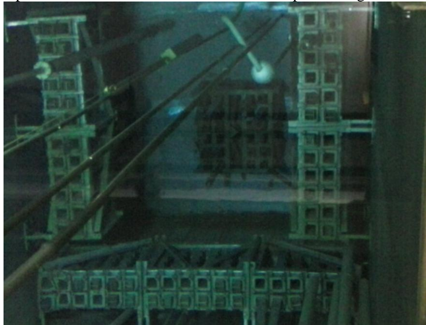
Figure 1: Current photo of the racks for spent fuel elements of the IEA-R1.
