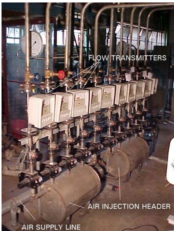
Fig. 6: Air injection Header and Air injection lines.
