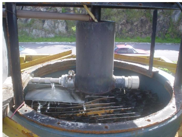
Figure 3. Photo of motorized distributor apparatus.
