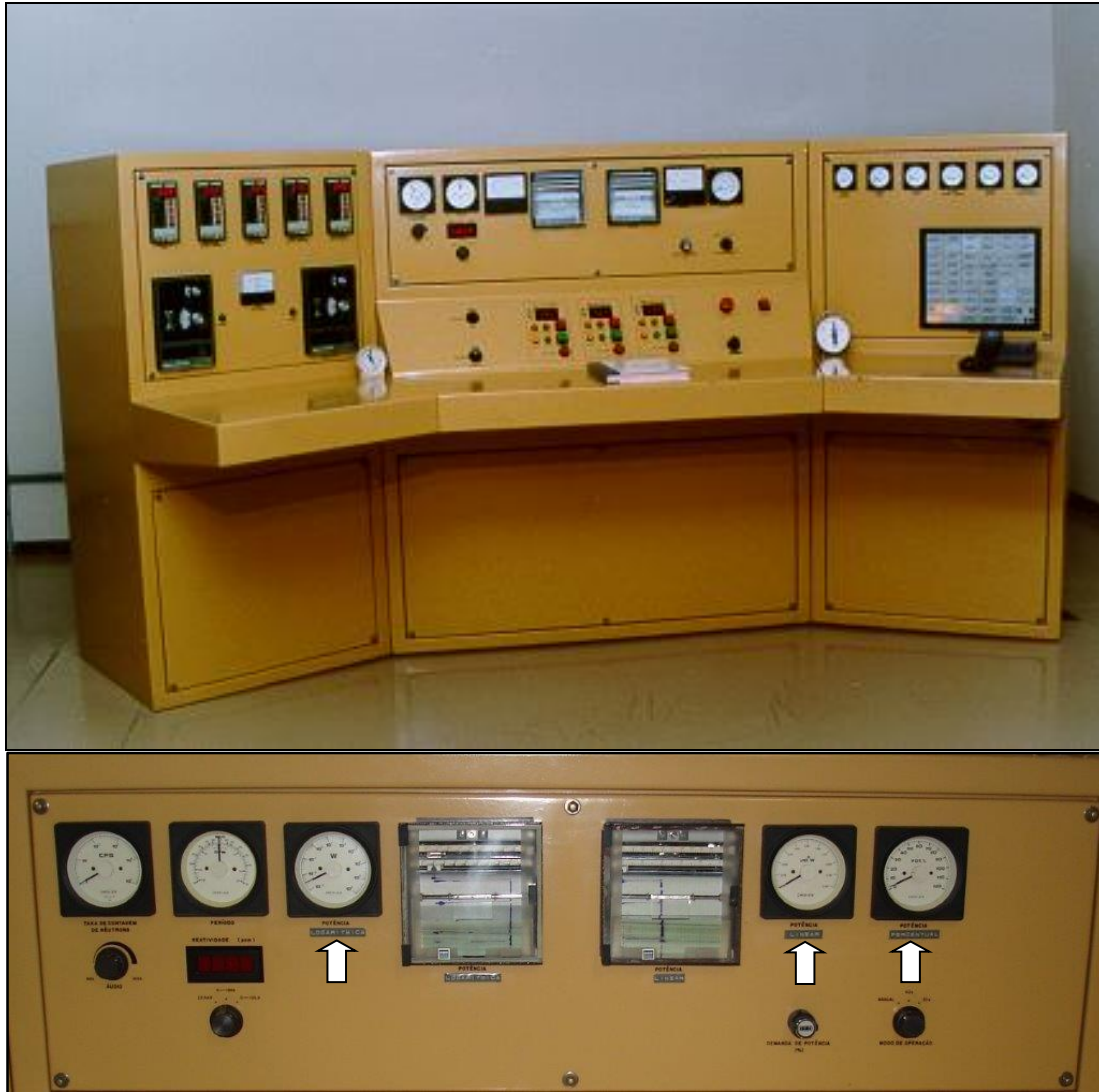
Figure 2: Top: IPR-R1 control console. Bottom: details of IPR-R1 control console; from left to right, arrows indicate Log N, Linear and Percent Power Channels.
