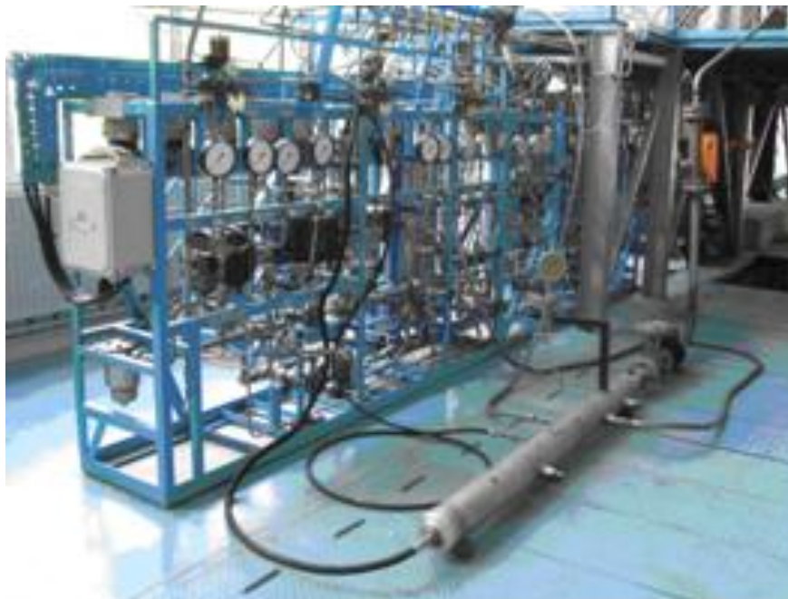
Figure 8 The Mechanical Simulator installed at the valve station
