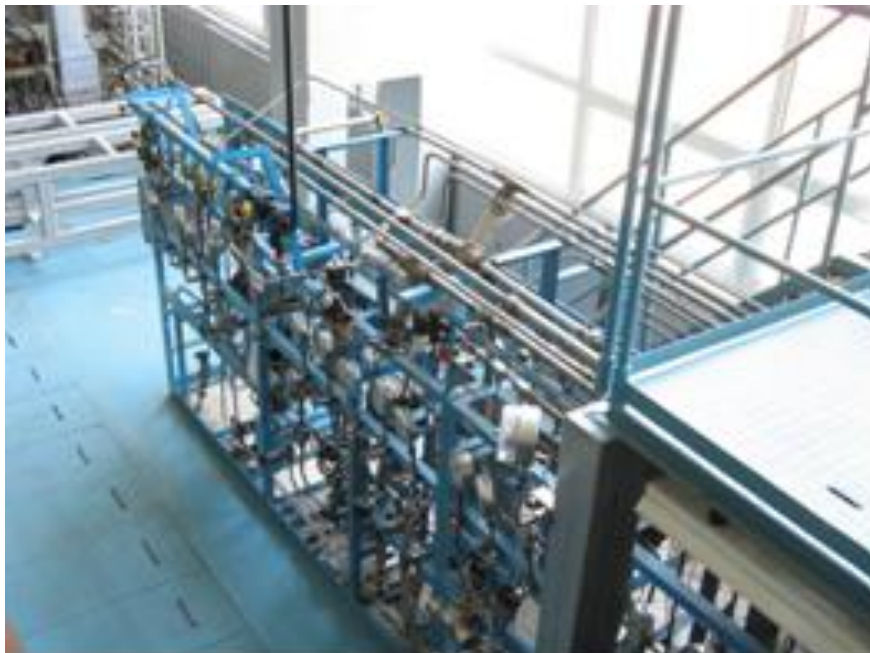
Figure 3 F/M testing rig: valve station (partial view)
