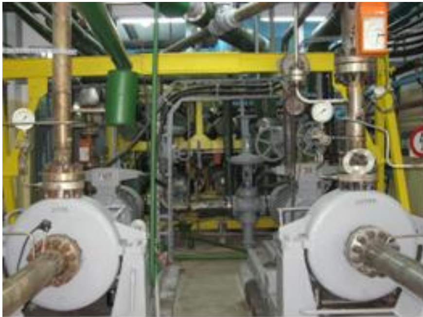
Figure 2 F/M testing rig: thermo-mechanical loops (partial view)
