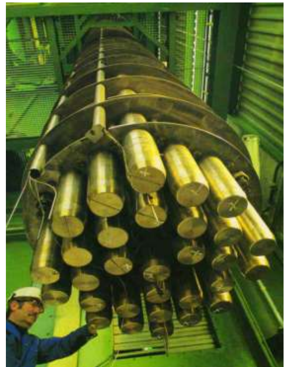
Fig 2: Photo of Tube Bundle of the “Helium heated Reformer, REF”. Look from the entry side of high temperature Helium of 950°C upwards in the direction of the helium flow, guided by baffles. This baffle-bundle was tested first. Later the double-tube bundle was also tested.
